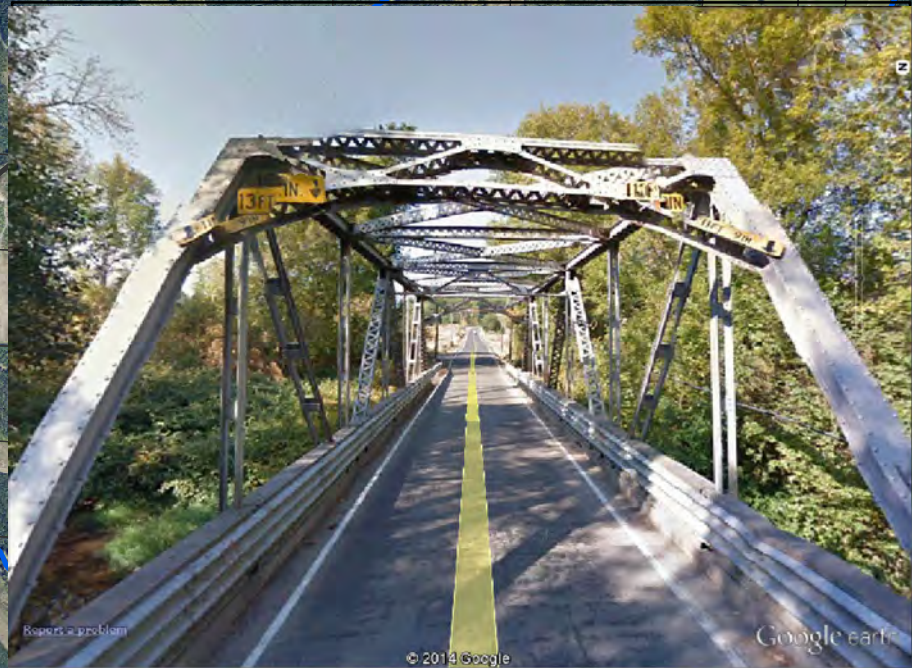
The Ferrier Bridge #93 is a steel truss bridge which was initially erected in 1924 and rebuilt in 1988.
